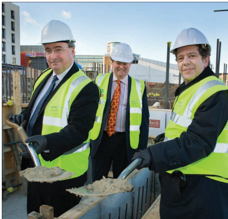
Above: Patrick McGhee, Vice-Chancellor of UEL, Mark Stevens, Chair of UEL's Governors, and Master of Birkbeck David Latchman pour the first cement at the new building in Stratford (Geoff Wilson)
