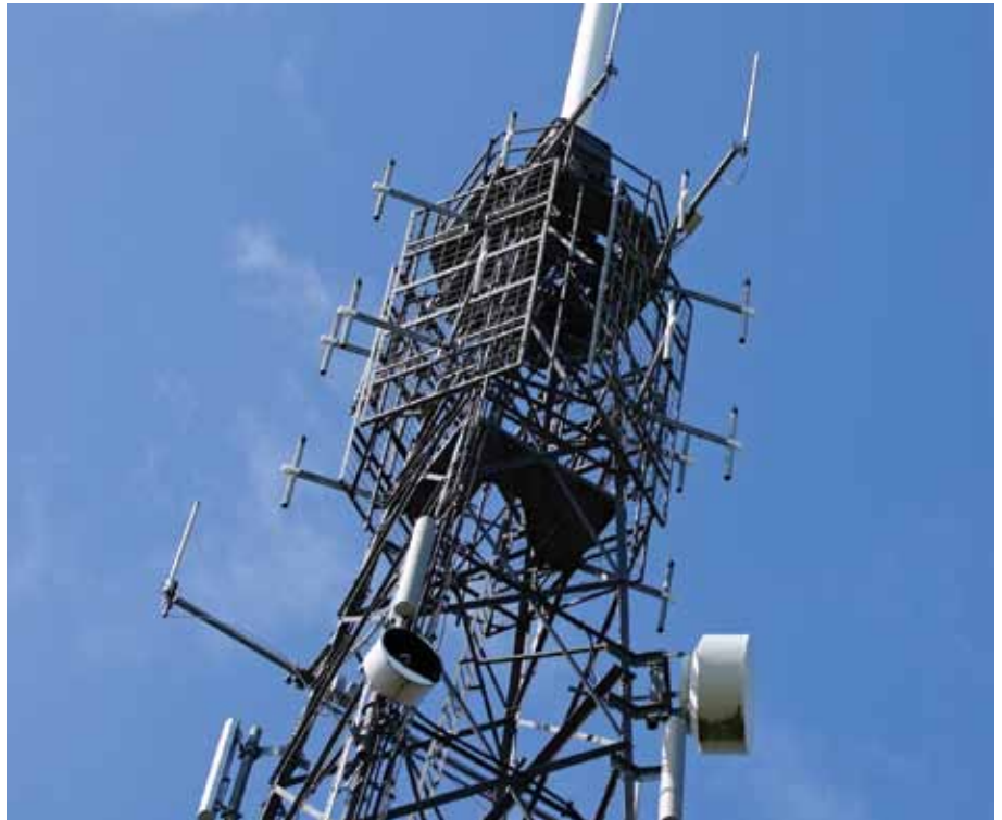
Multi-use telecommunications towers are a cost effective way of providing UHF and VHF broadcast, GSM mobile phone connectivity and point to point microwave links. A key aspect of this provision is the correct frequency allocation and interference suppression circuitry studied in the MSc in Wireless Systems.
